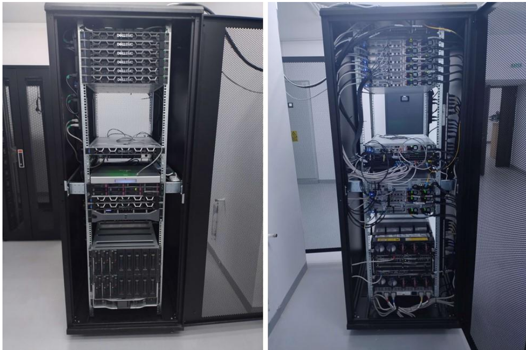
Fig. 20-6 Sistem High Performance Computing (HPC).
